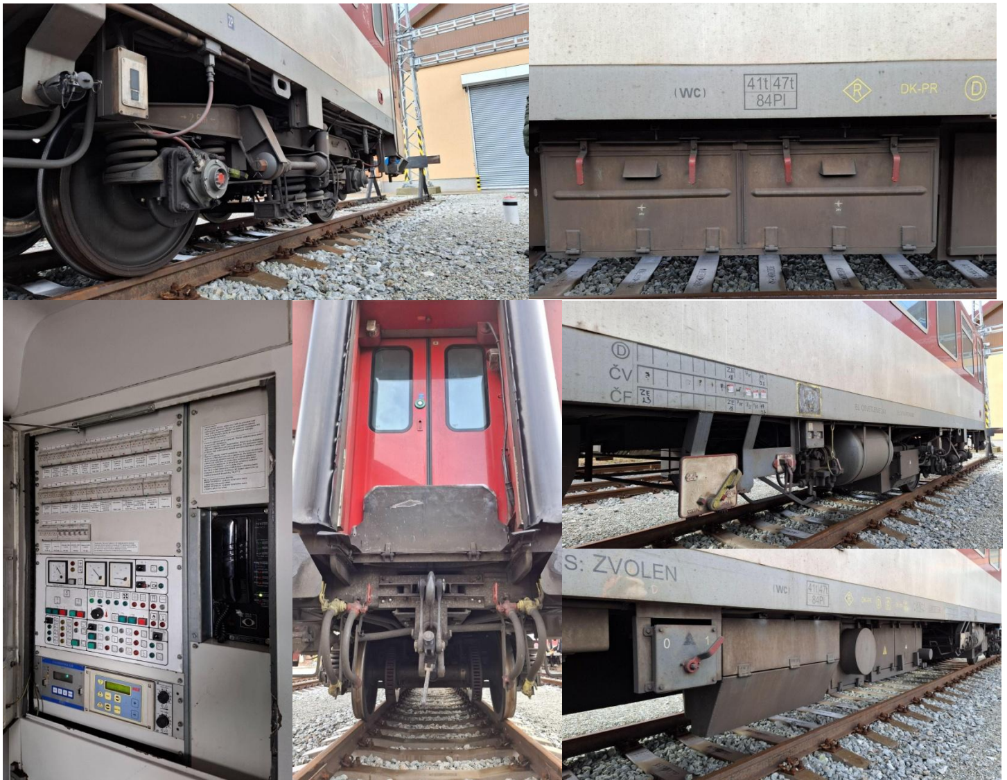
Pic. No. 11 A look at the outdated solution of unclosed cabinets
